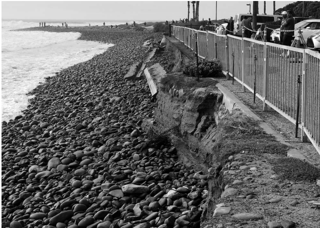
Figure 11. Erosion of the bike path and bluff along the Promenade in Ventura California during the large wave event of January 9th, 2019.
