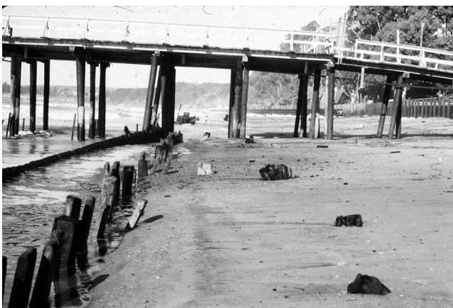
Figure 7. Timber and sheet pile bulkheads have been built and destroyed nine times over the past 86 y.
