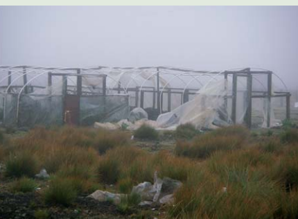
FIGURE 3 Greenhouse construction was funded in an effort to motivate smallholders to grow more vegetables for home consumption, thus improving family nutrition. This is an example of a recent development project (which appeared to be successful a couple of years ago) in the highlands that began with good intentions but has since been abandoned by both the development agency and participants (Photo by Matthew Taylor).
