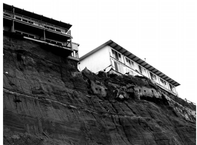
Figure 13. These apartment buildings in Pacifica were built on a high eroding bluff in the early 1970s, and despite efforts to protect them, they were declared unsafe to occupy and then demolished in 2016.
