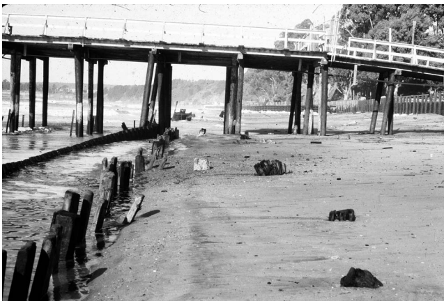
Figure 7. Timber and sheet pile bulkheads have been built and destroyed nine times over the past 86 y.
