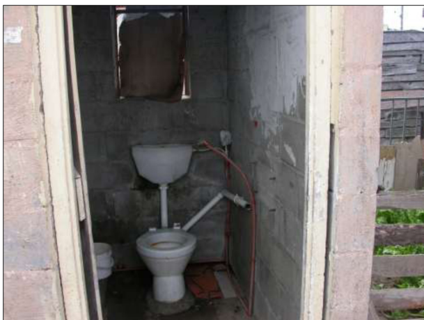
Figure 5. Tap against the wall on right is either lost or removed. Note the broken pipe and cistern, as well as the broken window which has been repaired with cardboard in Masipumelela.
