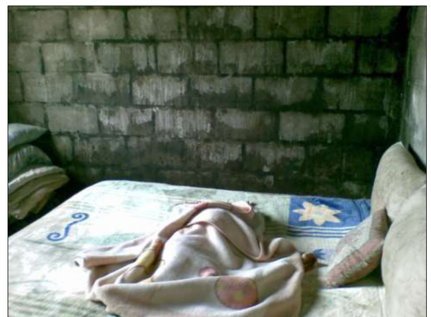
Figure 3. Dampness penetrating bedroom wall with infant sleeping on bed in a low-cost house in Greenfields.
