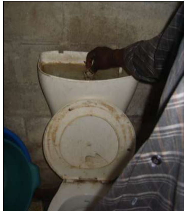
Figure 6. Flushing mechanism on this toilet is broken in a house in Masipumelela. Users flush toilet by manually manipulating the mechanism inside the system. Note that the toilet is dirty.
