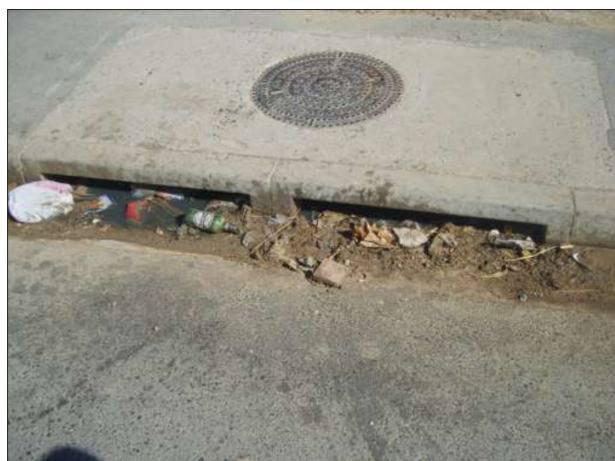
Figure 8. Solid waste blocking the storm water inlet on street causing subsequent flooding during rain storms in Greenfields.
