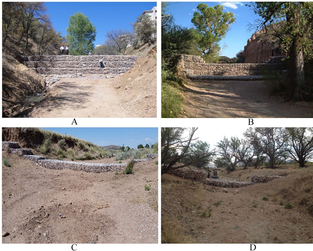
Figure 4. (A) Looking downstream at Cinco de Febrero, which experiences major flooding during monsoons, in Nogales, Sonora, Mexico (photo by Hans Huth [April 12, 2010]); (B) Gabion in Hay Hollow at Rancho San Bernardino, Sonora, Mexico (by Josiah Austin [October 27, 2001]) 67 ; (C) Gabion in Vaughn Canyon on the Babacomari Ranch (by James Callegary June 19, 2015); and (D) Gabion installed at Bone Creek on the Deep Dirt Farm Institute (by Kate Tirion (2014). See Figure 3 for map locations.
